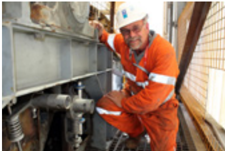
Simple modifications to the export conveyor system at the Kwinana Bulk Terminal have improved safety and product handling, and reduced cleaning costs and environmental impact.
