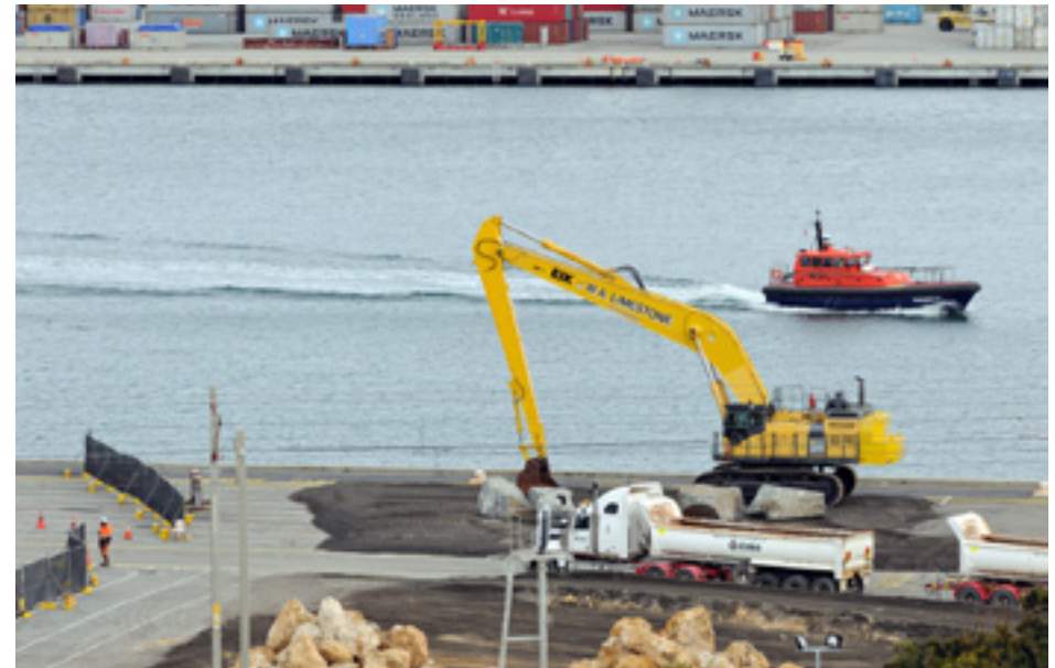
Stockpiling rocks at J Berth, Victoria Quay in preparation for construction of an underwater rock mound to protect the Fremantle Rail Bridge
